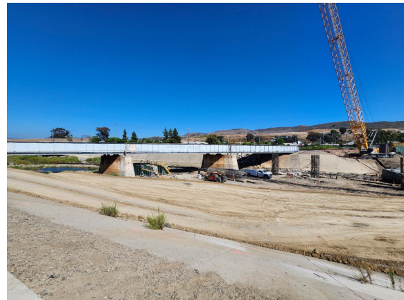
Site clearance and preparation for abutment work near San Juan Creek Trail.
