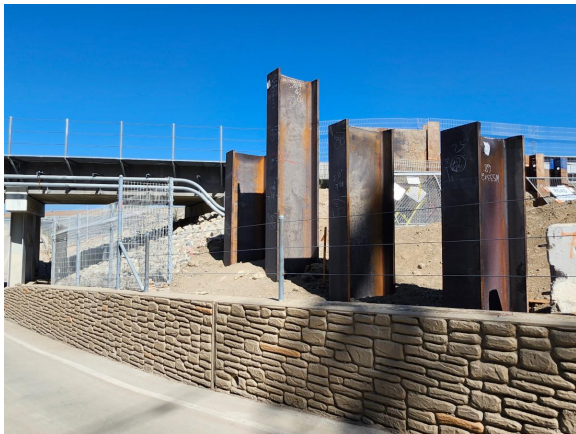
Piles, also referred to as steel beams, installed by crews in early August.
