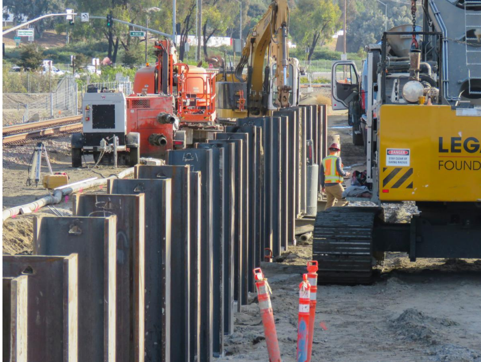
A row of installed steel piles for one of four retaining walls.
