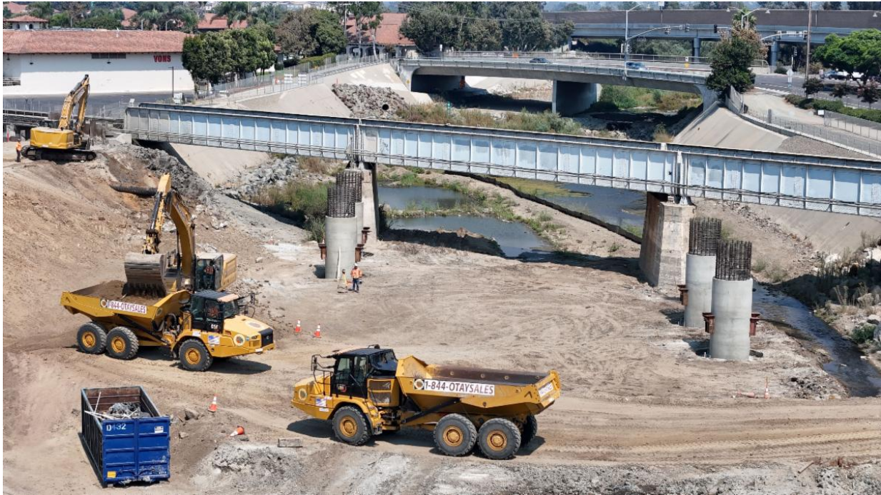
Four concrete piers, or bridge supports, installed to support the new rail bridge.
