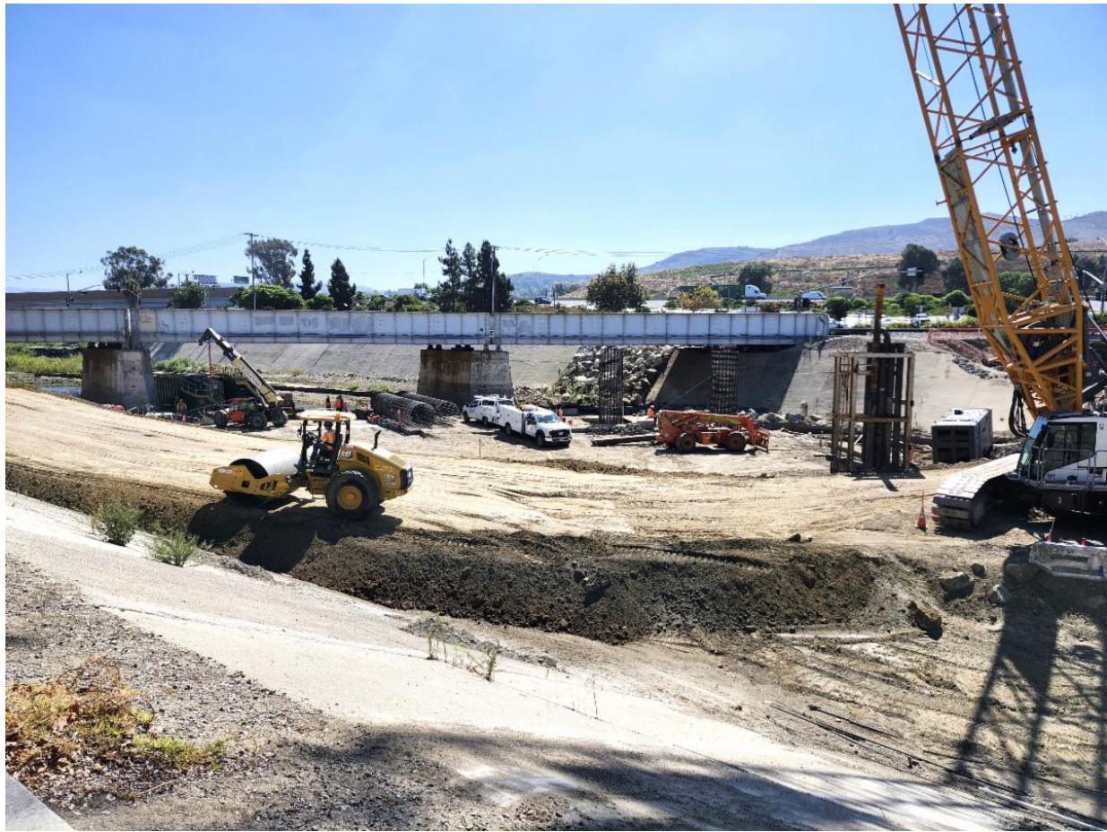
New access ramp built near the trail as crew prepare to construct an abutment near the trail.
