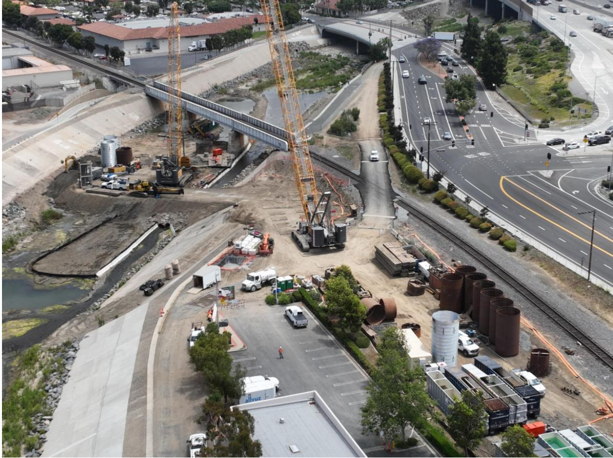
View of project site and staging area in preparation for construction of the bridge foundation. Activity seen in the photo is the installation of metal pipes.
