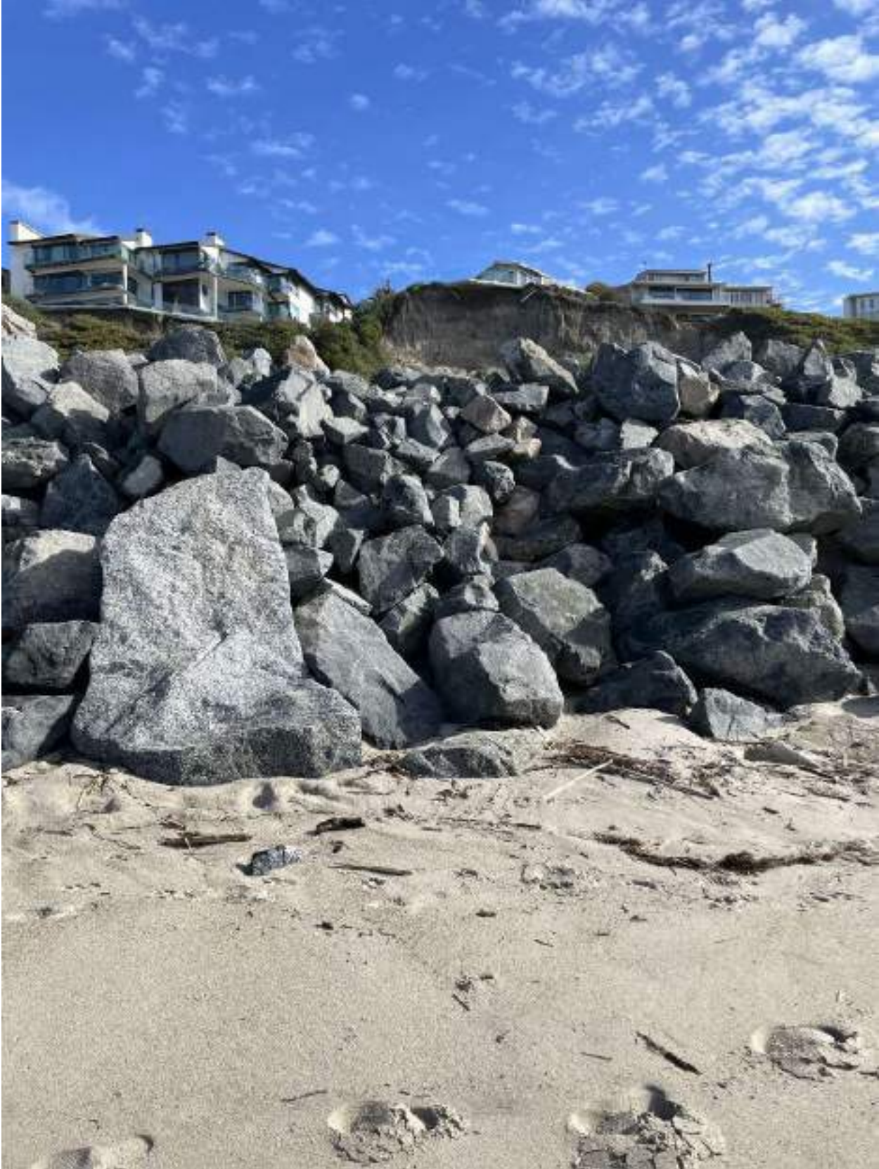
Figure 9 – Undersized and oversteep rock in southern repair area
