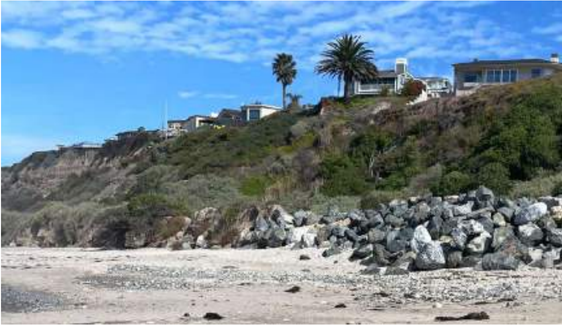
Figure 7 – Transition From Proposed Riprap Repair to Southern End of Proposed Engineered Revetment
