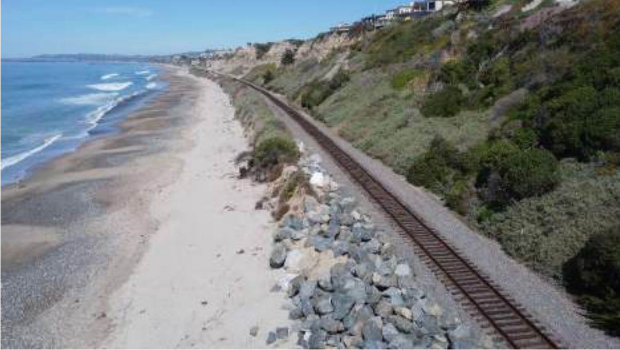
Figure 2 – Proposed Southern End Of New Engineered Revetment Where Vegetation Ends and Rock Begins
