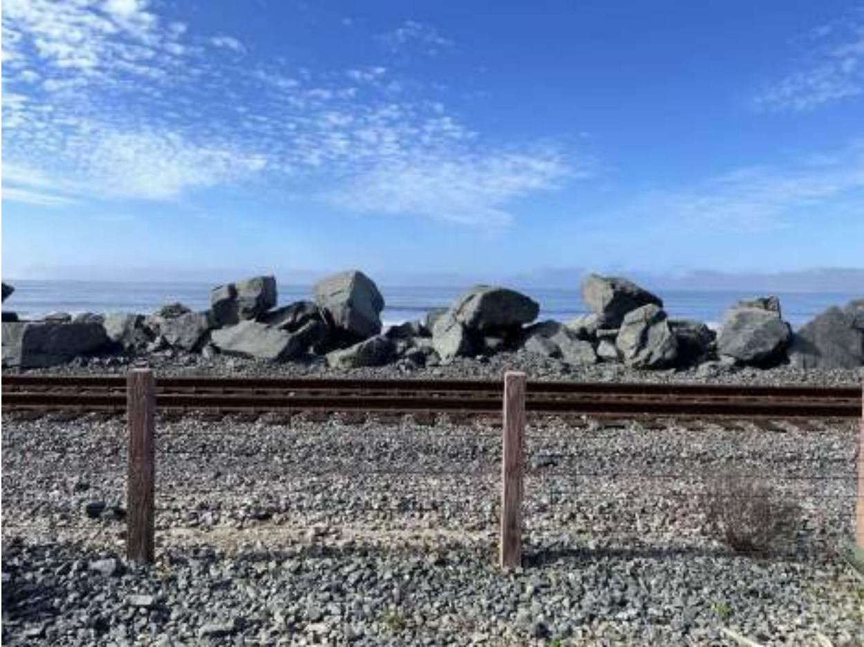
Figure 10 – Riprap crest showing stones with inadequate points of contact with other stones
