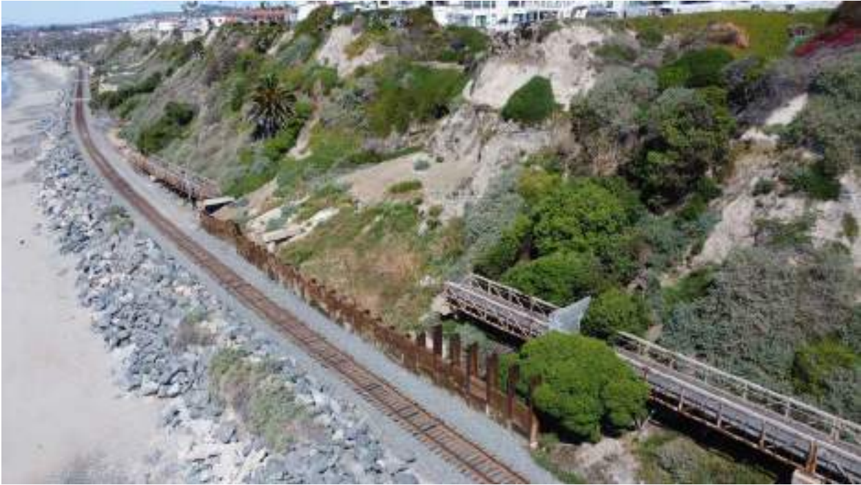
Figure 3 – Recent Bluff Failures at MP 204.2 (Mariposa Pedestrian Bridge)
