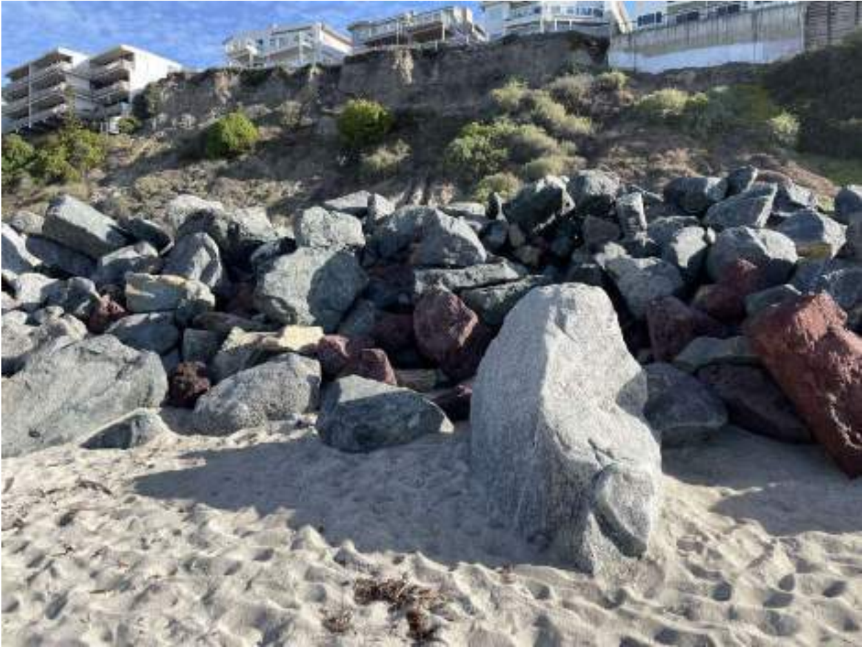
Figure 1 – Typical current site conditions at north end of repair area viewed from high beach berm
