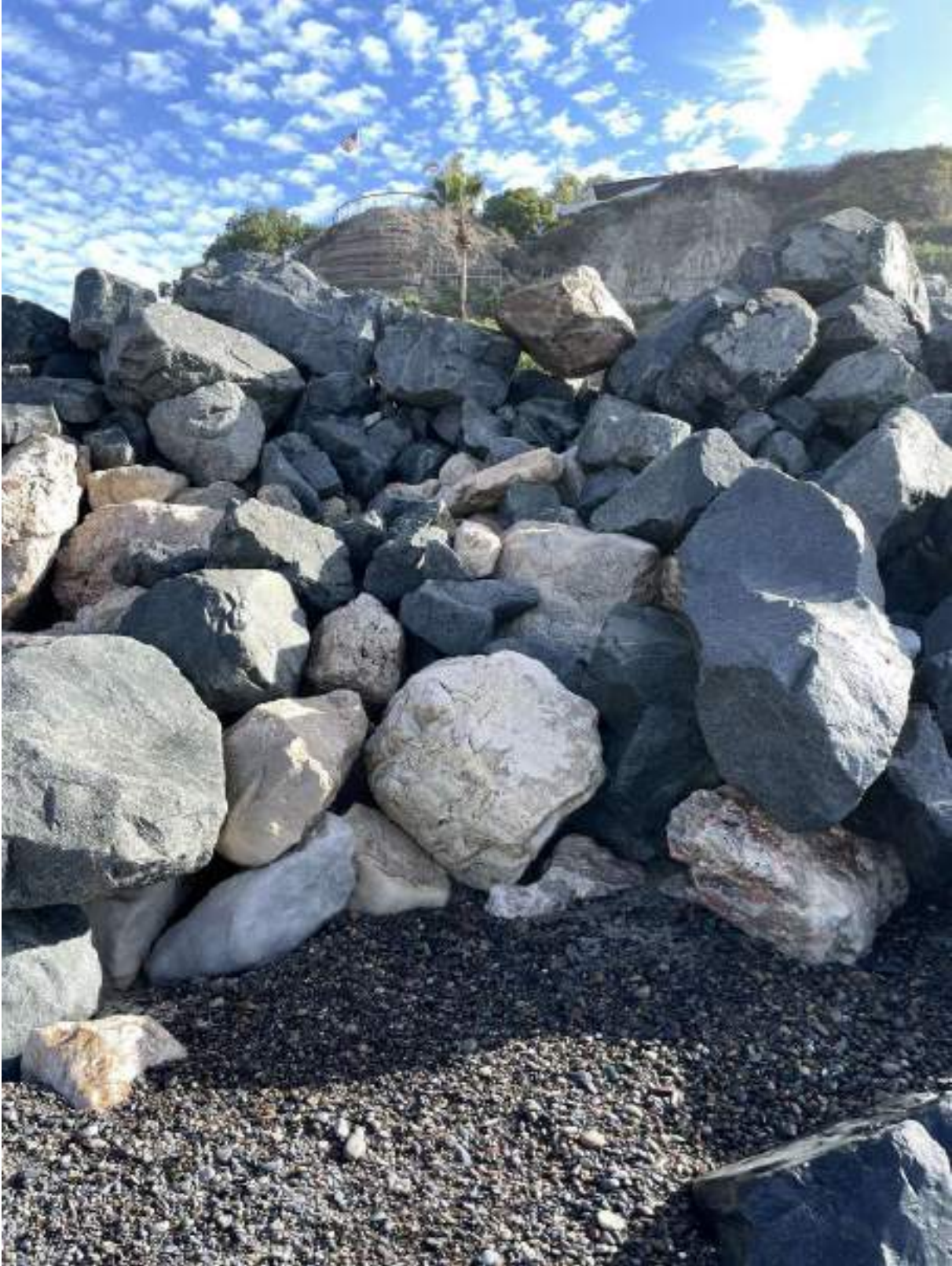
Figure 4 – Undersized stones and unstable stones at crest
