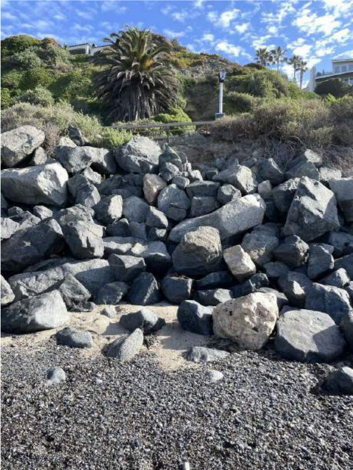
Figure 6 – Undersized and displaced stones and exposed natural embankment at south end of repair area
