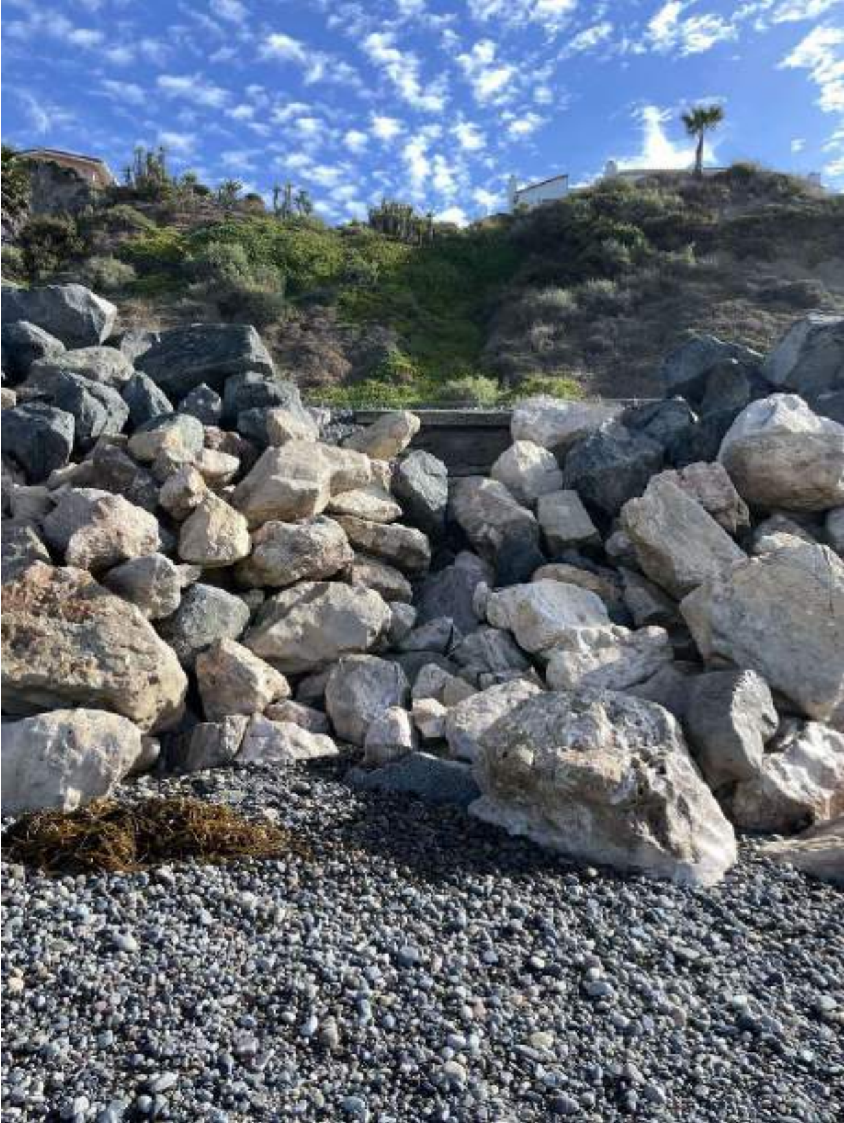
Figure 5 – Undersized stones, exposed ballast and no crest protection at culvert outfall
