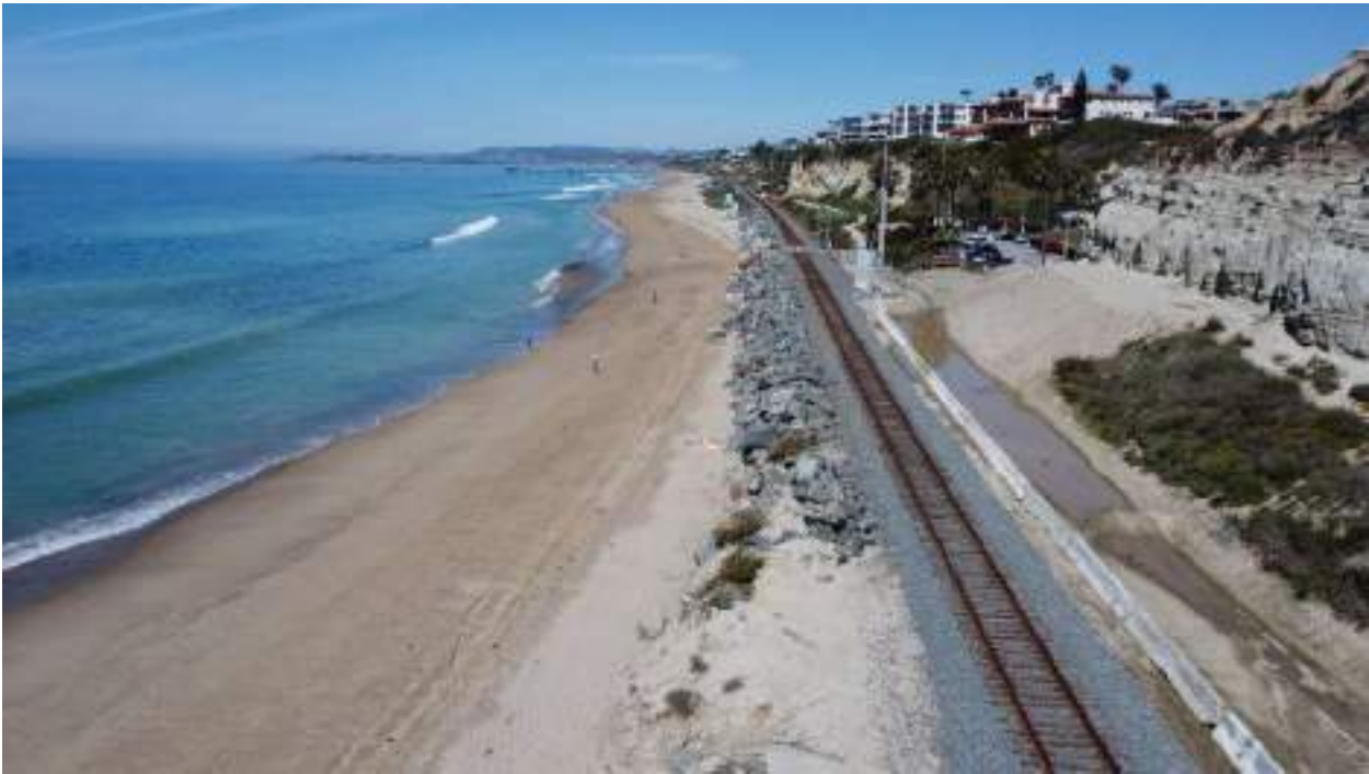
Figure 5 – Proposed North Riprap Repair Area Near MP 206.10
