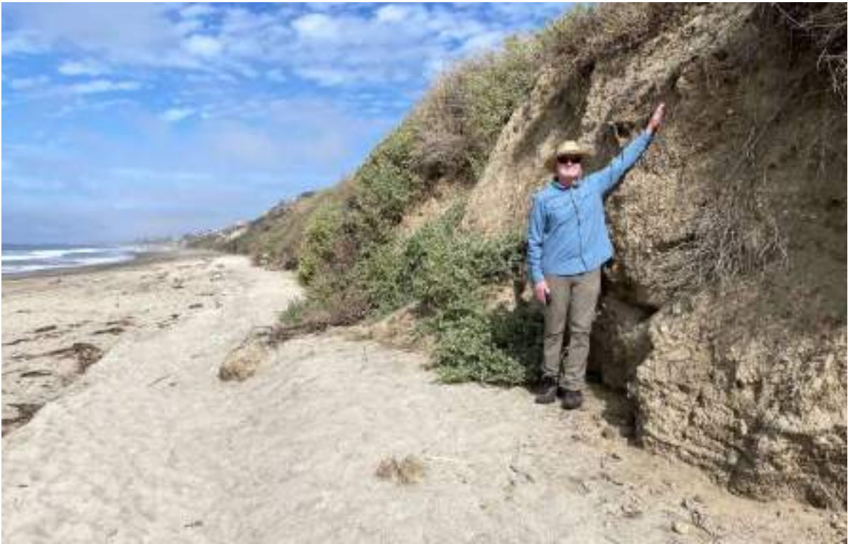
Figure 9 - Existing Eroded Berm at Southern End of Proposed New Engineered Revetment
