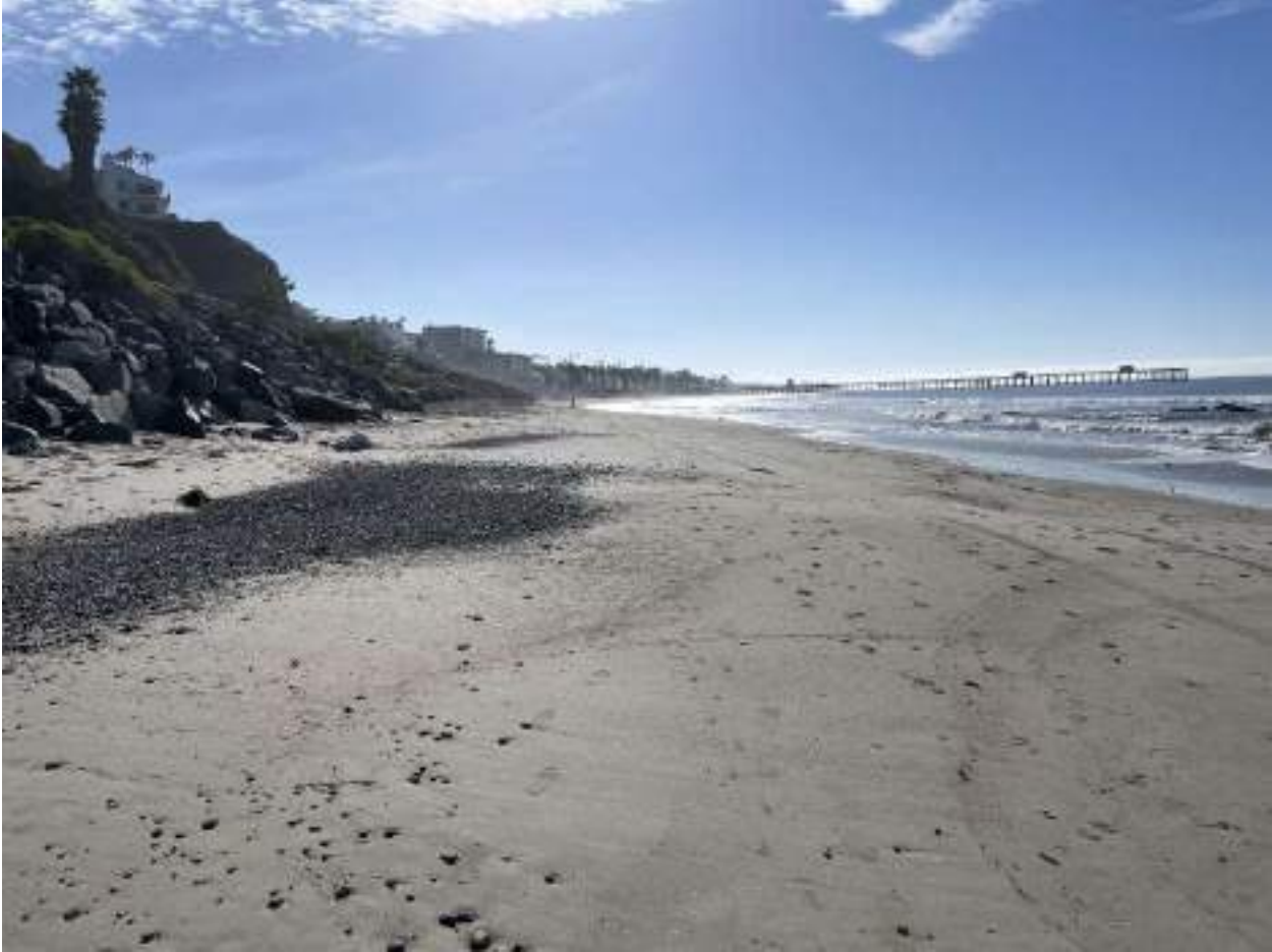
Figure 8 – Existing beach condition at low tide facing southeast, at southern end of repair area
