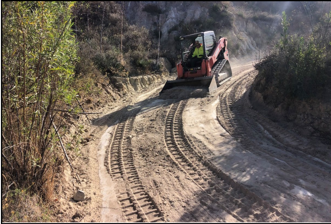
PHOTOGRAPH 14 Recontouring of Fire Road in Rose Canyon to Repair Erosion Ruts and Rills, Trabuco Rose Preserve, November 2023
