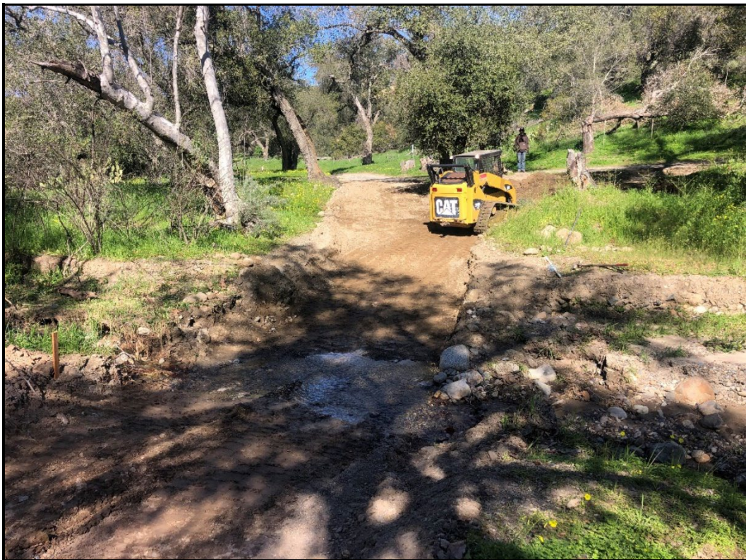
PHOTOGRAPH 2 Apex Repairing Easement Road Where It Crosses Hickey Creek, Trabuco Rose Preserve, January 2023
