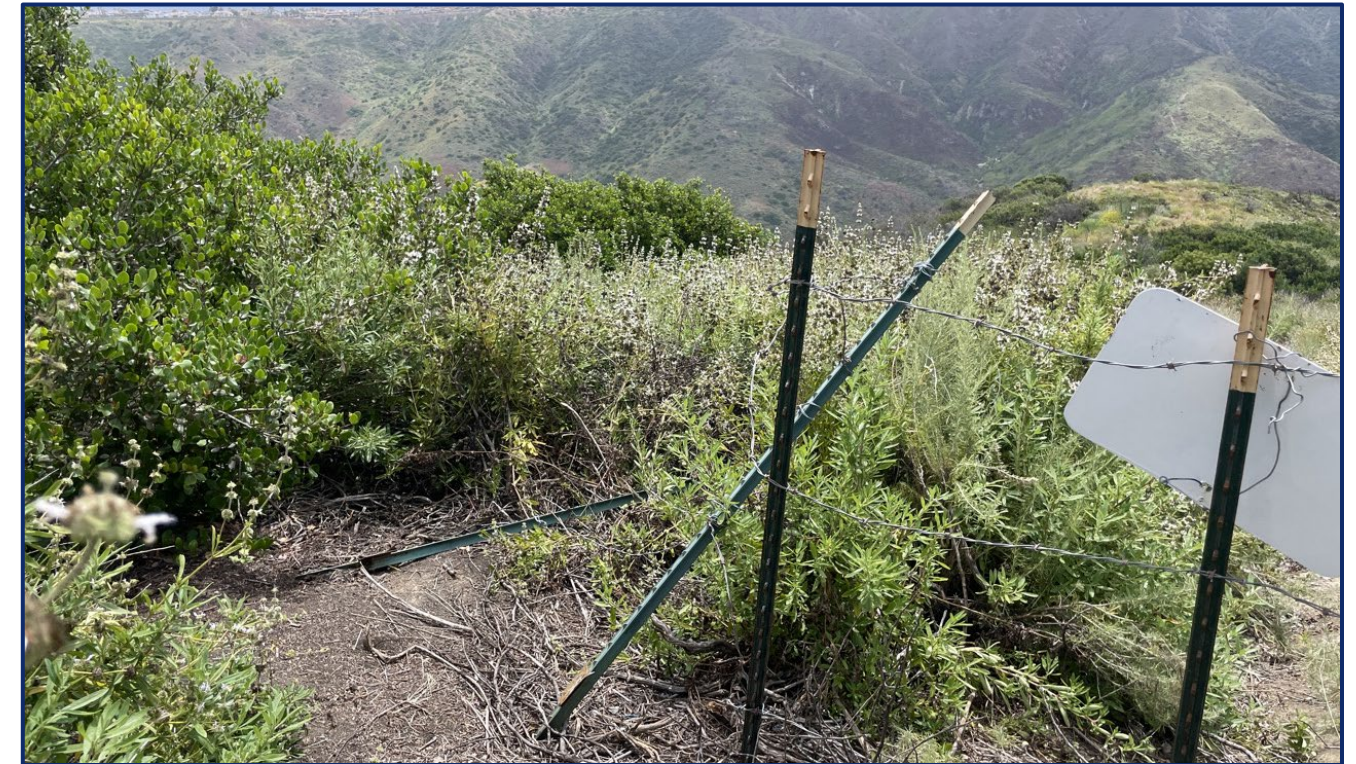
Photograph 8: Depicting fence in need of repair. Photo taken June 22, 2023.
