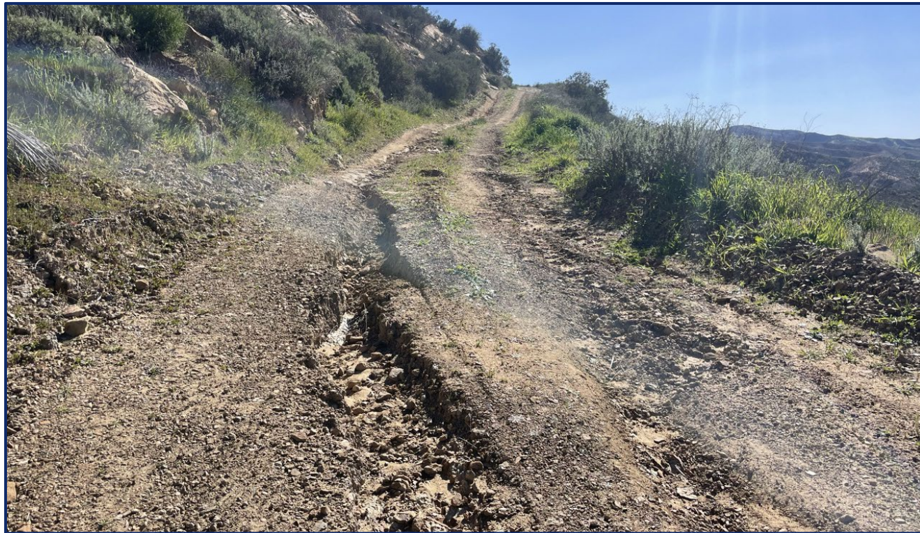
Photograph 5: Depicting deep erosion on main access road. Photo taken February 15, 2023.
