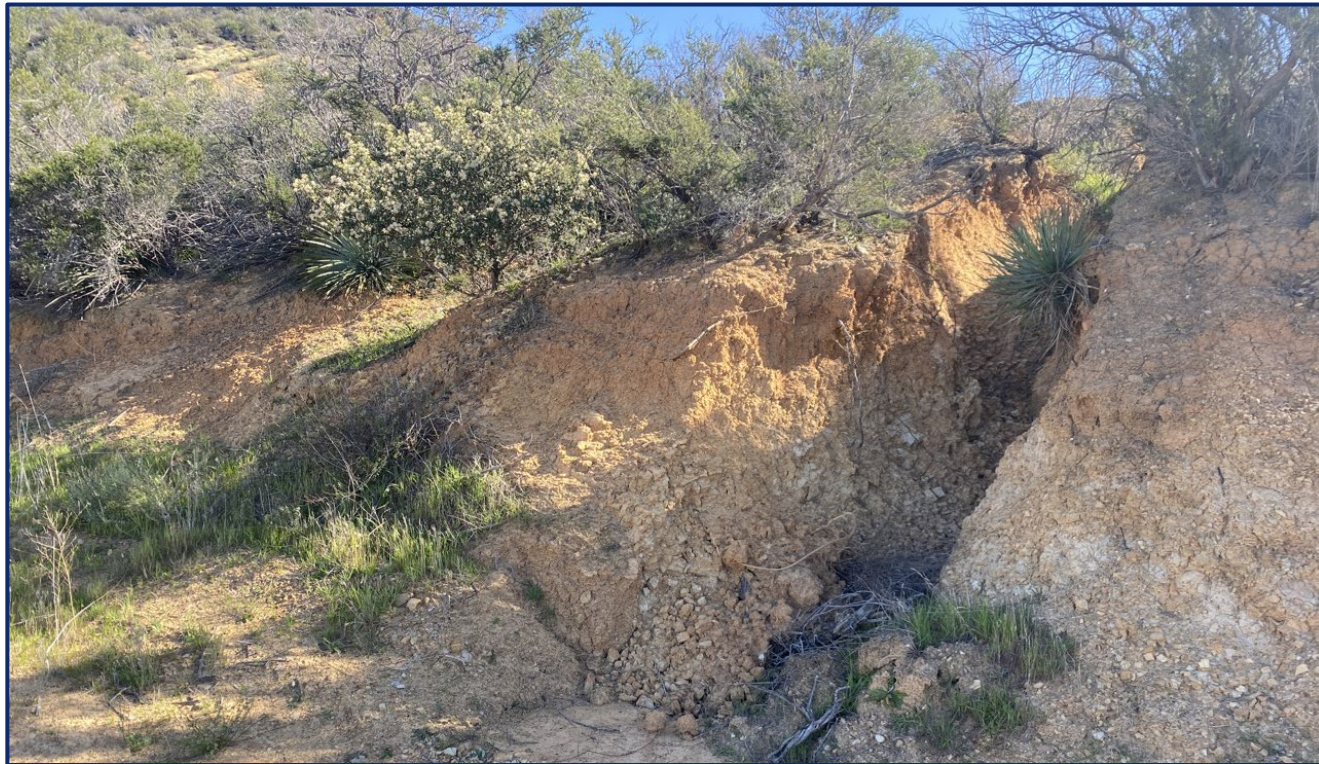
Photograph 3: Depicting erosion cutting across trail. Photo taken February 15, 2023.
