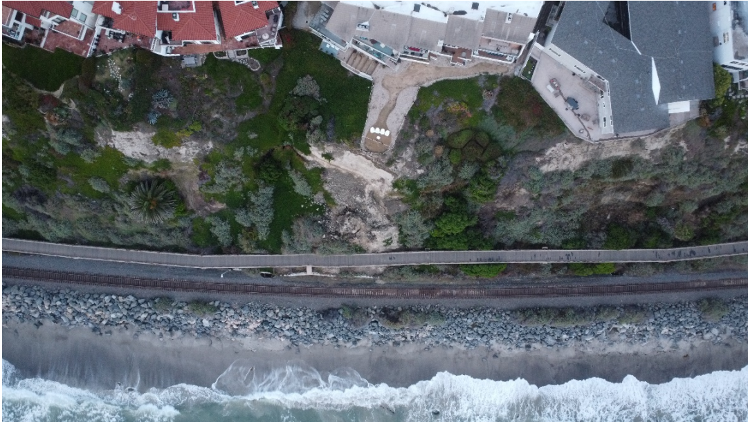
Figure 15. Potential Reinforcement Site 3: MP 204.00 to 204.50, steep bluffs, potential to impact tracks, poor track-side drainage with potential for liquefaction – January 21, 2024
