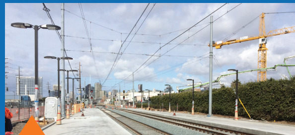
Wires going across the road. This wire arrangement will be used in sections of the alignment where the streetcar travels in both directions.
