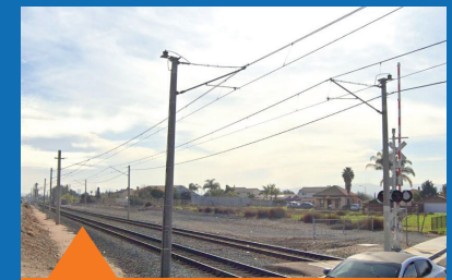
Wires between vertical poles. Wire will be strung between poles on the same side of the road for all other sections of the alignment.
